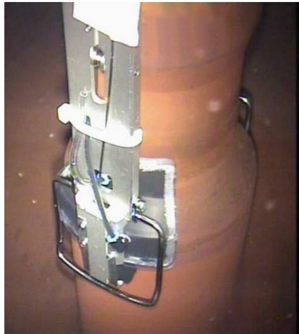
MouldMan tooling applied on emergency nozzle during A-VT inspection for defect height sizing.
